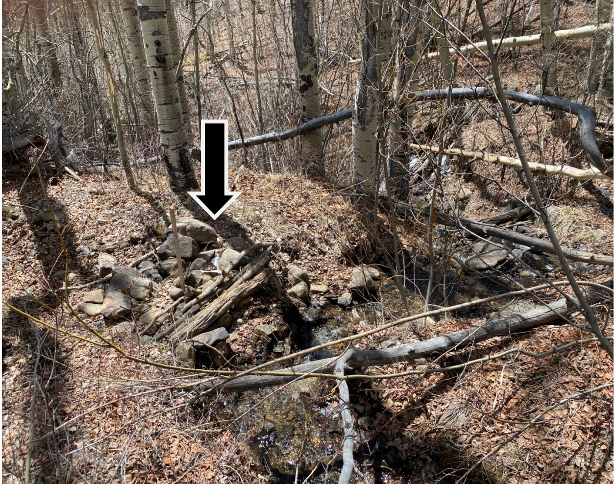
Looking south just below 1 st dam at DWR 2 nd dam (black arrow), plugging the east fork on the left. West fork is on the right where all the water from Bartlett Gulch is now flowing.
